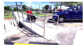
Six ramps have been constructed in Tropicana LSI following the MS 1188-2014 Malaysian standard as part of MPSI's Barrier Free City pilot project for the benefit of disabled pedestrians. — Fpaz
